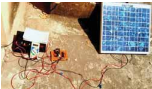
Fig. 15 Hardware setup of the system
